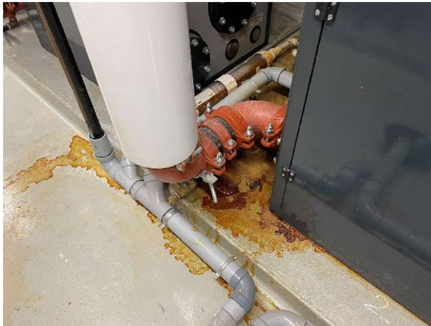
Photograph 44 – Interior, boiler room Looking at unknown stains located in the boiler room floor.
