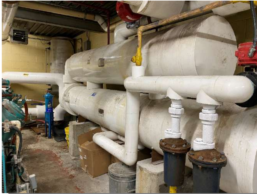
Photograph 37 – Interior, ammonia tanks Looking at ammonia tanks stored to the north of the Arena.
