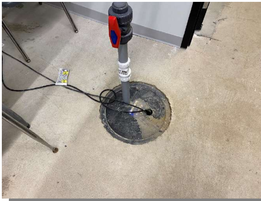
Photograph 42 – Interior, drain Looking at a drain located in the basement storage room.
