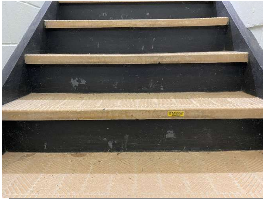
Photograph 43 – Interior, stairs leading to the second floor Looking at potentially asbestos containing materials on the stairs leading to the second floor.
