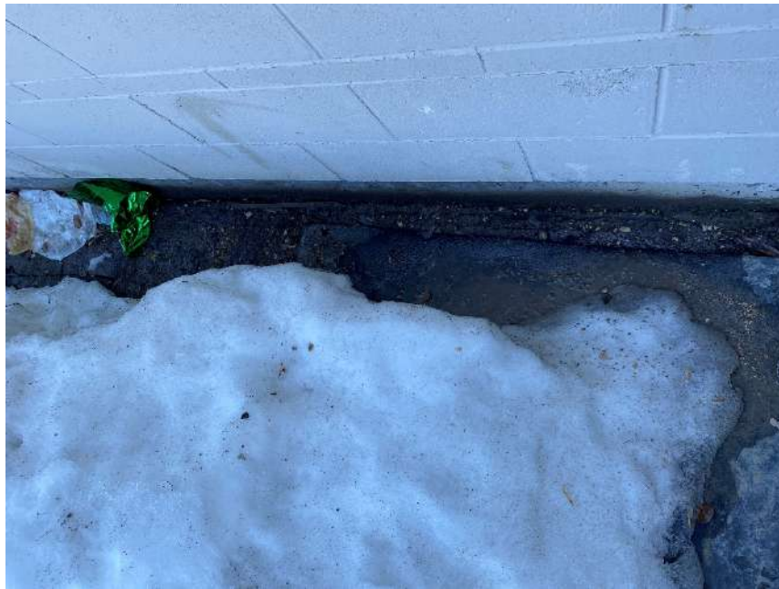
Photograph 38 – Exterior, oil contamination Looking along the northwest corner of the building at oil contamination that has not been cleaned up.
