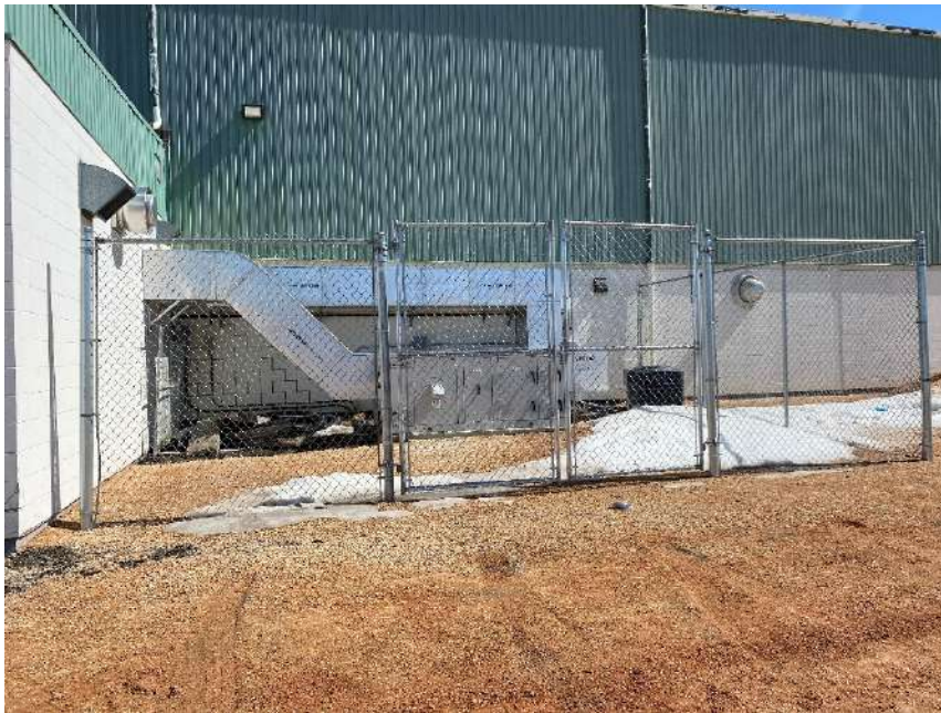
Photograph 40 – Exterior, air handling unit
