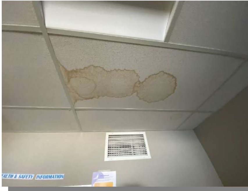
Photograph 41 – Interior, ceiling stain Looking at water damage stains on the ceiling of the staff kitchen that is to be removed.
